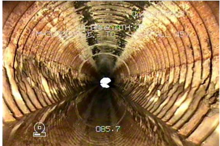
Figure 6: CSP Internal Corrosion
