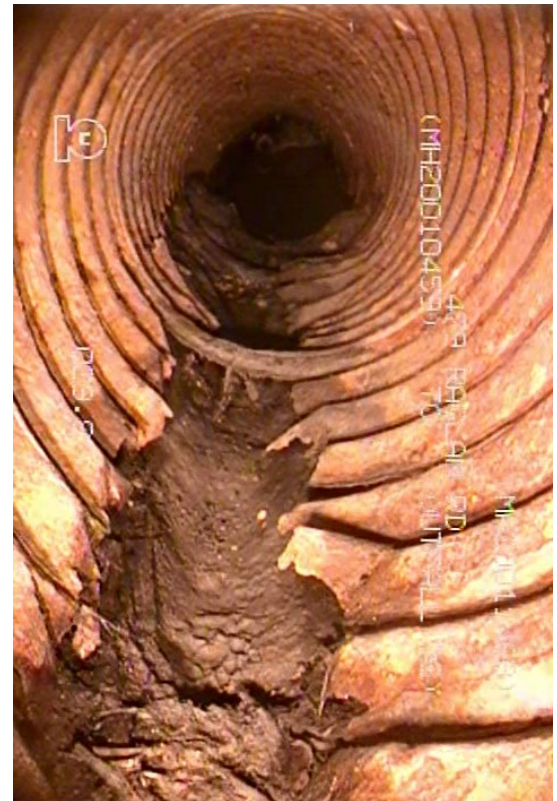
Figure 23: Missing invert within CMP
