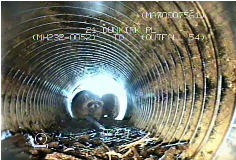
Figure 22: Raccoon Nesting Within Degraded CMP Outfalls
